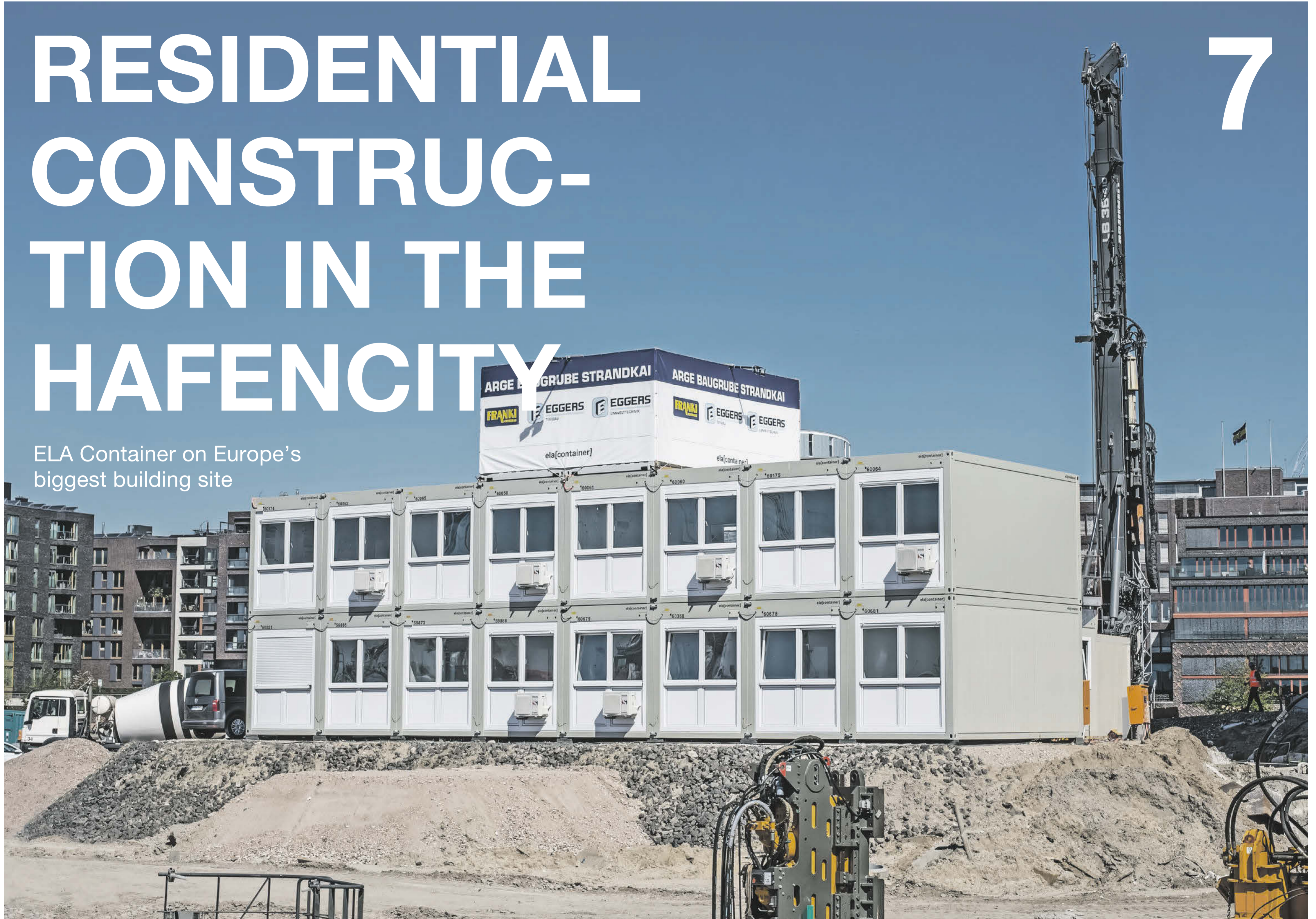
A planner's eye view: the ELA building site facility on Hamburg's Strandkai.
